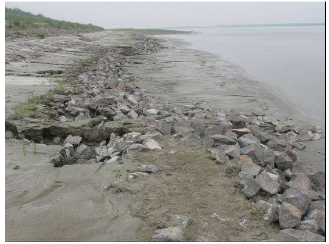
(b) Damaged section with shifted rock with exposed geotextile and some sand deposits
