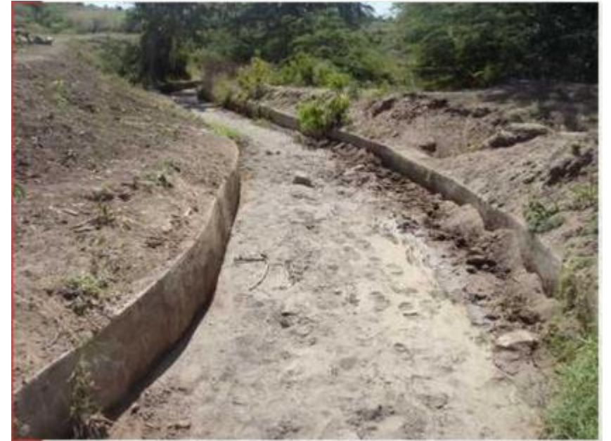
Canal filled with sediment
