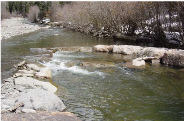
Figure 11-29 Cross vane structure with step on the East Fork Piedra River, CO
