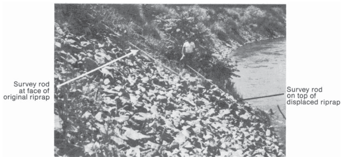
Figure 3.69. Damaged riprap on left bank of Pinole Creek at Pinole, California, following flood of January 4, 1982.
