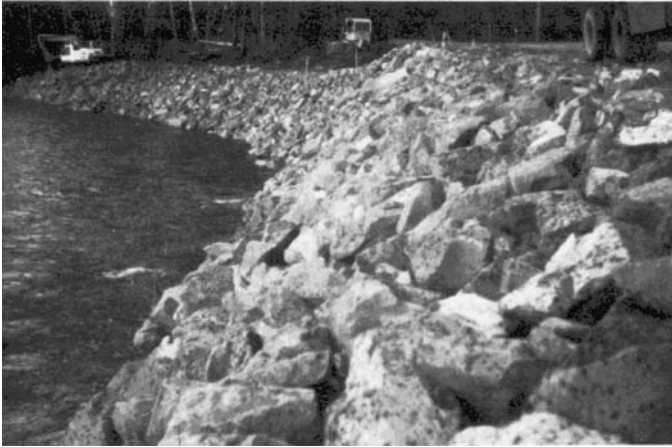
Riprap was damaged by modified slump at a location near truck tires during flooding in autumn of 1982 (photographed before failure August 1982).
