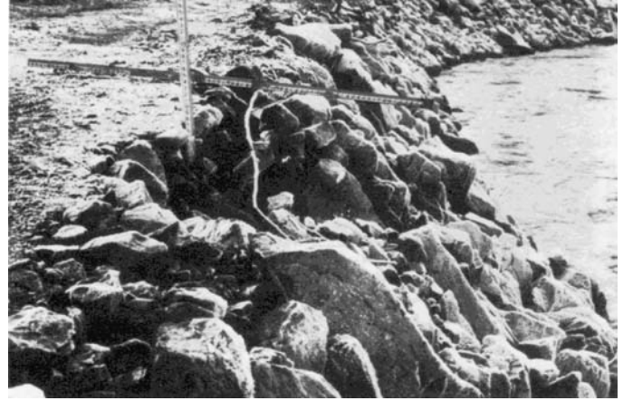
Damage is attributed to particle erosion by impinging flows that overtopped bank during flood of December 3, 1982 (photographed December 1982).
