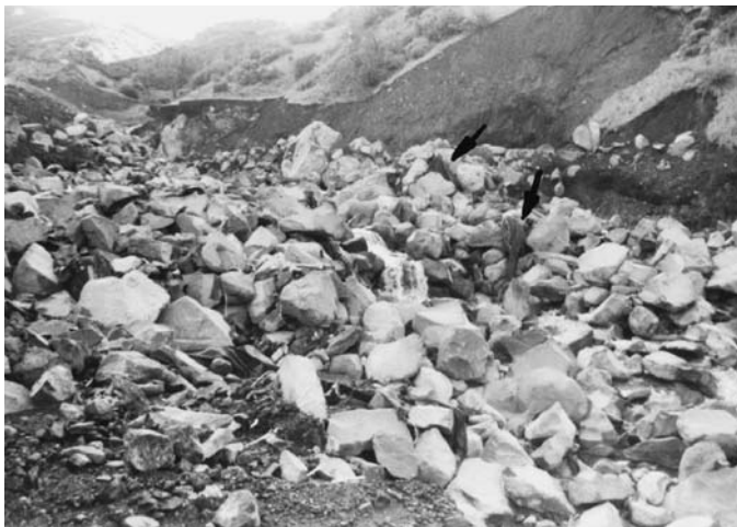
View is looking upstream. Woven-tape geotextile (slit-film) marked with arrows is inappropriate as RSP-fabric on banks (photographed May 1995)
