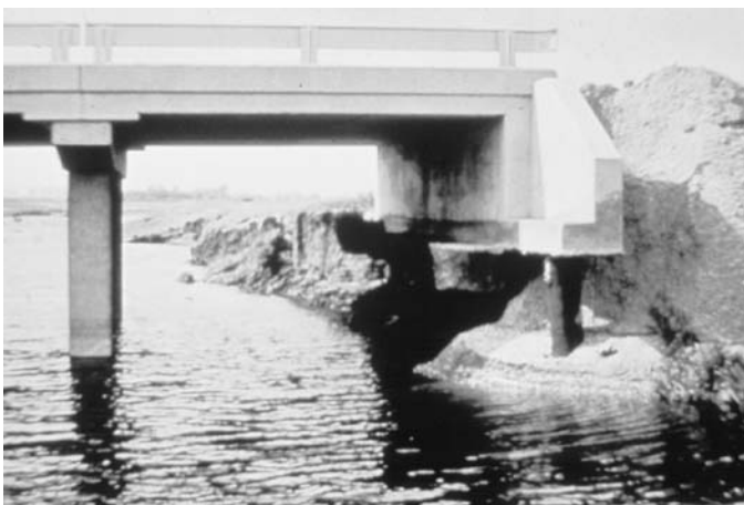
Figure 2.6. Scour of bridge abutment and approach embankment.
