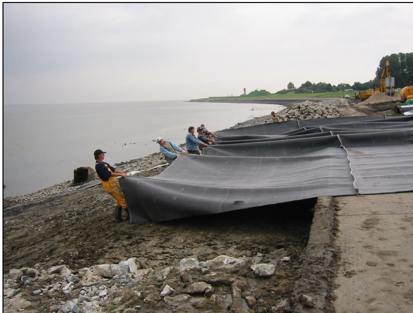
Figure 12.17. Hand placing geotextile prior to placing partially grouted riprap. Note sewn seam.
