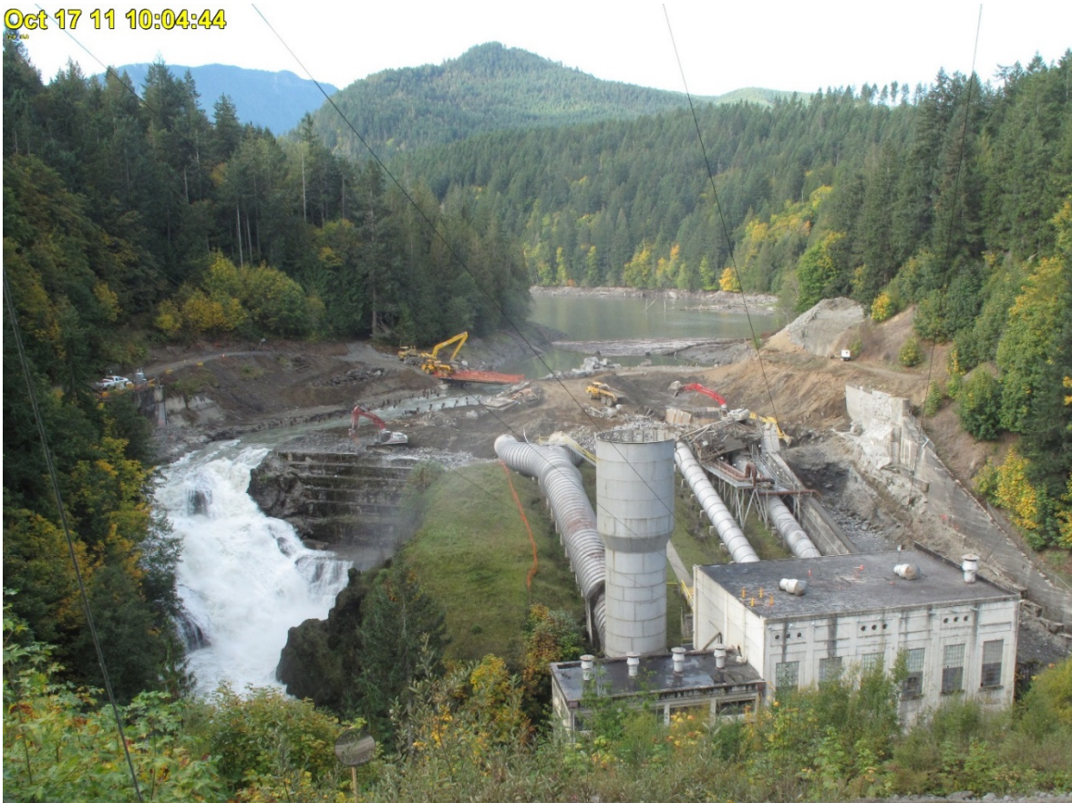
Figure 31.—Photograph of Lake Aldwell spilling through an excavated breach in Elwha Dam near Port Angeles, WA on October 17, 2011.
