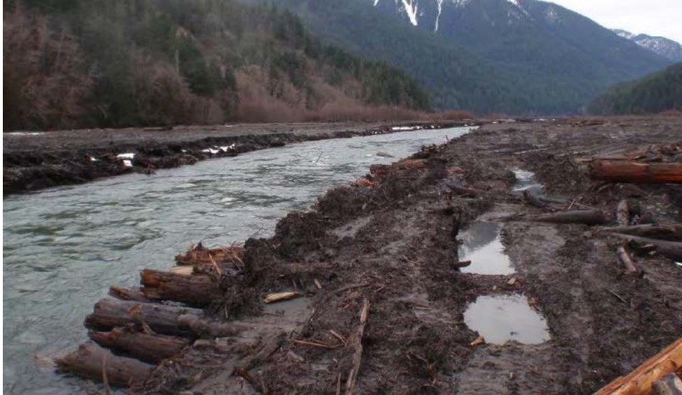
Figure 23.—A pilot channel excavated through the Lake Mills delta and alder forest growing on the delta was cleared in preparation for the removal of Glines Canyon Dam near Port Angeles, Washington (photograph courtesy of Bureau of Reclamation, December 2010).
