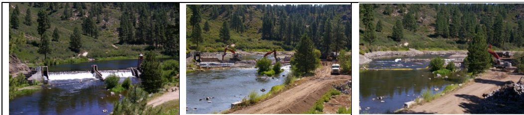
Figure 33.—Chiloquin Dam on the Sprague River just prior to dam removal in 2008 (left), during dam removal in 2008 (center), and after dam removal in 2008 (right).
