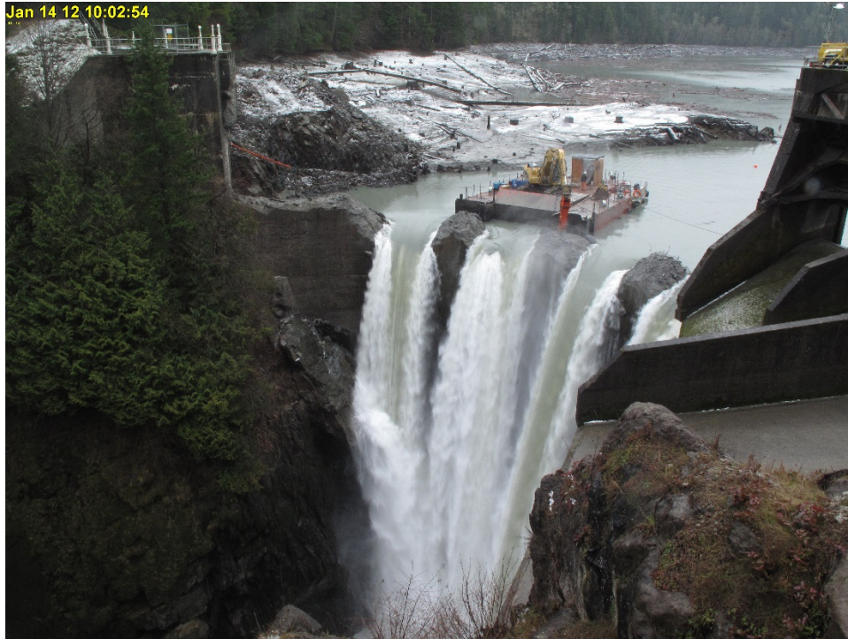
Figure 21.—A series of notches were cut into Glines Canyon Dam (near Port Angeles, WA) with a hydraulic hammer to release river flows downstream during dam removal.
