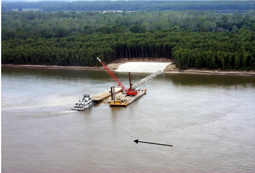
FIGURE 5.8 Dike Bank Paving On The Lower Mississippi River
