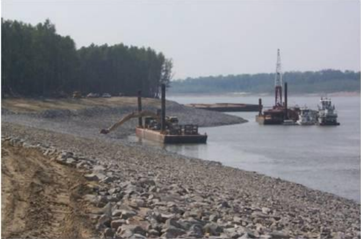
FIGURE 4.2 Stone revetment protecting a Mississippi River bankline
