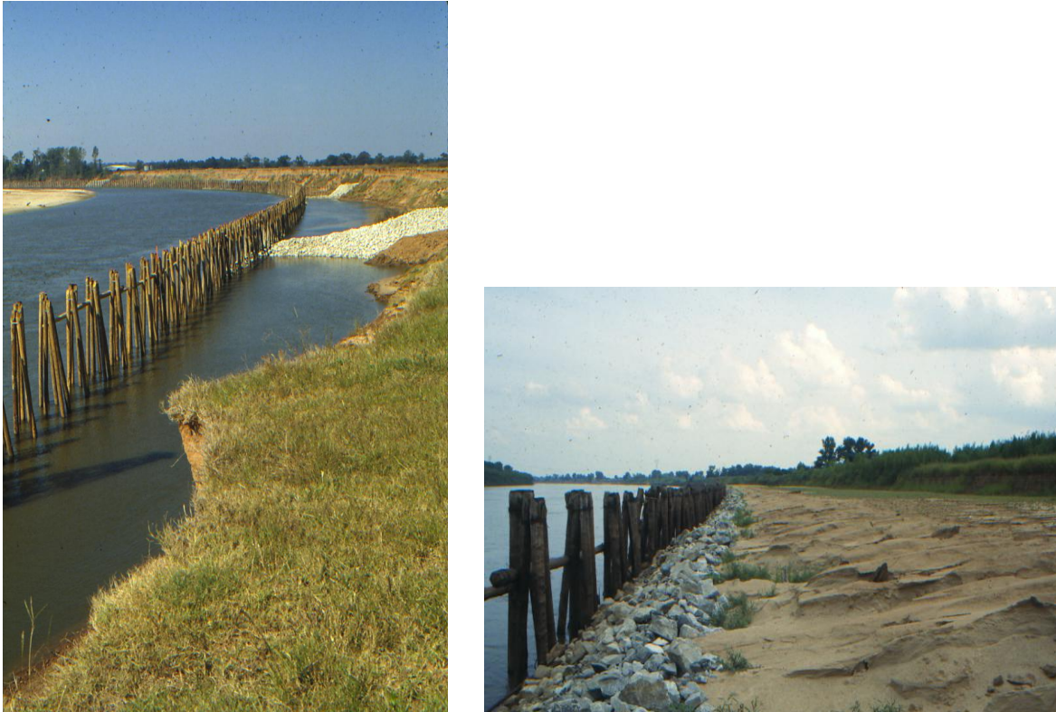
FIGURE 6.4 Photographs of Red River in Louisiana pile revetments – Immediately after construction and after sediment deposition had occurred
