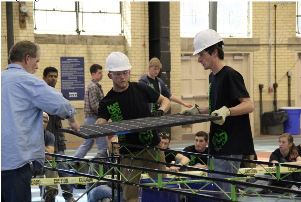
Placing the Decking Support Surface (Safety Steel Grating) at one location of the bridge from 2013.
