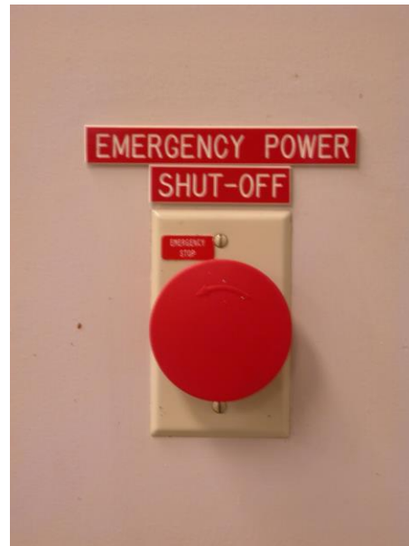
Switch on west wall above horizontal band saw.
