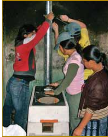
CSU seniors install a cookstove that they designed to replace fire pits used for cooking and heating in Guatemalan homes. The senior design team worked with a retired engineer and a service organization to speed stove production. There is a 10-year plan to produce 1.3 million new stoves, reducing indoor pollution and injuries to children.
