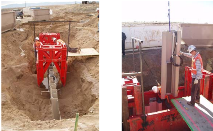
Figure 1. Installation of e-barrier through a plume containing RDX, 2,4,6-TNT, 2,4-DNT and 1,3,5-TNB
