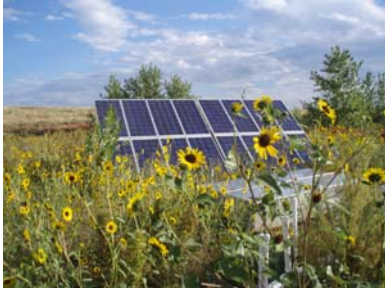
Figure 2. The e-barrier is powered by a 2 kW solar array consisting of 16 PV panels (BP Solar) and 3200 Ahr battery array (MK Battery). Voltage applied to the e-barrier is controlled using DC-DC converters (Vicor). Power consumption by the e-barrier is currently approximately 350 W.
