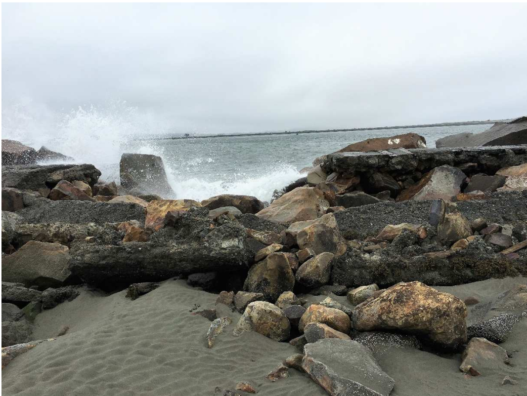
Figure 12 – Example of non-performance, armored coastal structure, Humboldt Jetties, Aug 2016. Photo by Patrick O'Brien
