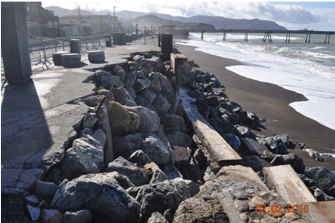
Figure 1 - Seawall failure, Pacifica, CA, winter 2015-2016. Photo by Patrick O'Brien
