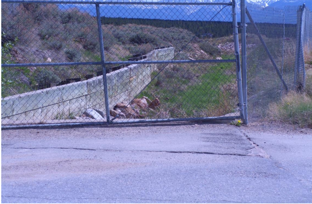
Figure C-65: Starr Ditch crossing at 3 rd Street. There is no flow in the channel—drainage flows away from the observation position toward California Gulch to the south.
