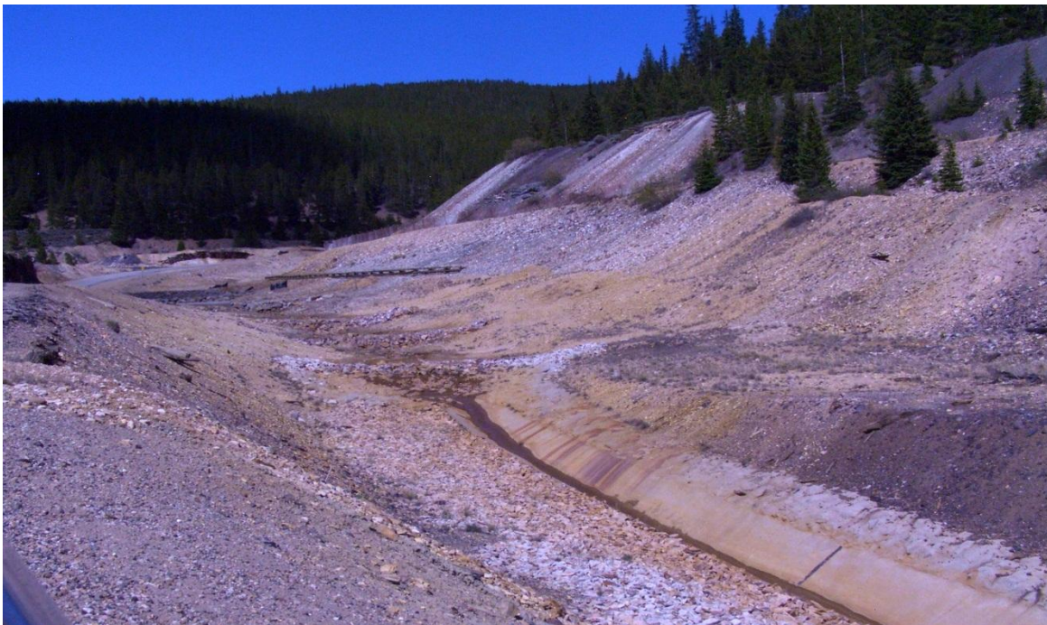
Figure C-4: Beginning of lined channel above CG-1. A series of five rock weirs is visible upstream of the lined channel.
