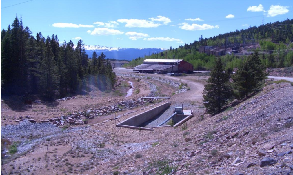
Figure C-7: View looking downstream at double channel in California Gulch near Yak Tunnel Portal below CG-1 gauge. Flow from the Yak Tunnel is collected from the left channel and delivered to the treatment plant approximately one-half mile downstream. Any flow from upper California Gulch (there is none in this photo) bypasses the treatment plant via the channel at right. Defunct flume is obscured but the foot bridge shows that its location is just upstream of the Yak ditch.
