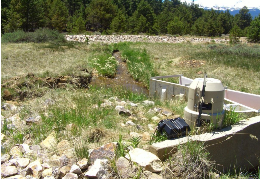
Figure C-37: Monitoring equipment on installed rip-rap on left bank with CG-5 flume.
