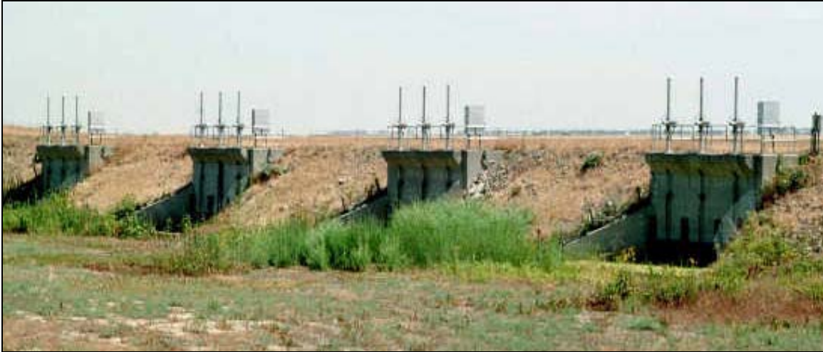
Figure 9: Front View of Inlet Gates Located at Gale Avenue
