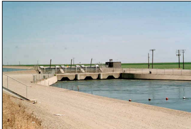
Figure 6: Radial Gates Located South of the Railroad Tracks along San Luis Canal
