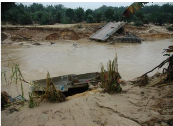
c) A bridge completely destroyed
