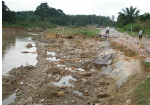
b) Eroded bank affected the adjacent road
