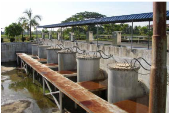
e) Pumping stations
