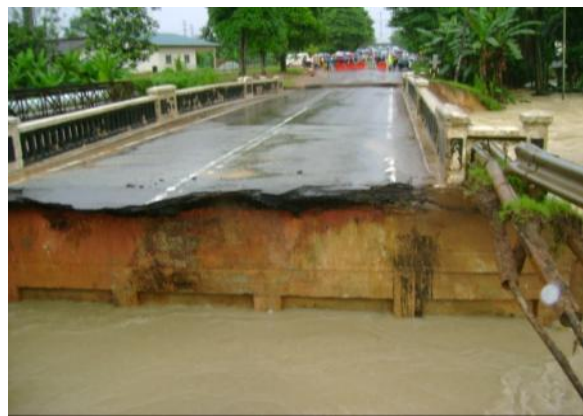
d) Another bridge also was swept away
