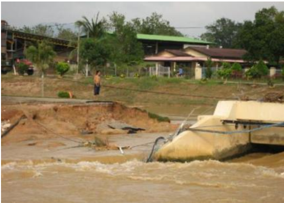
a) Flood wall swept away by the current
