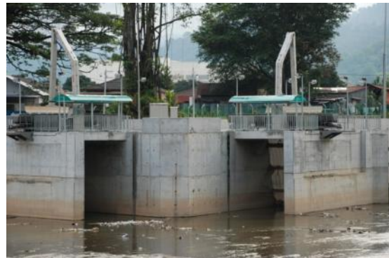
f) Debris removal system
