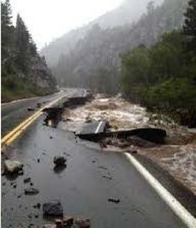
Road erosion and failure (2013, www.bizjournals.com )
