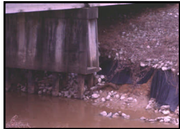
Damage to infrastructure due to bed degradation
