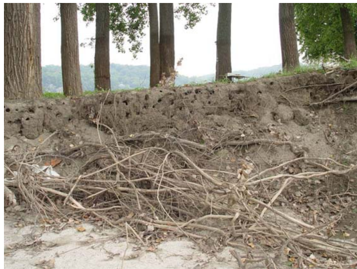
Figure 17. Root networks and crayfish tunnels throughout the levee.
