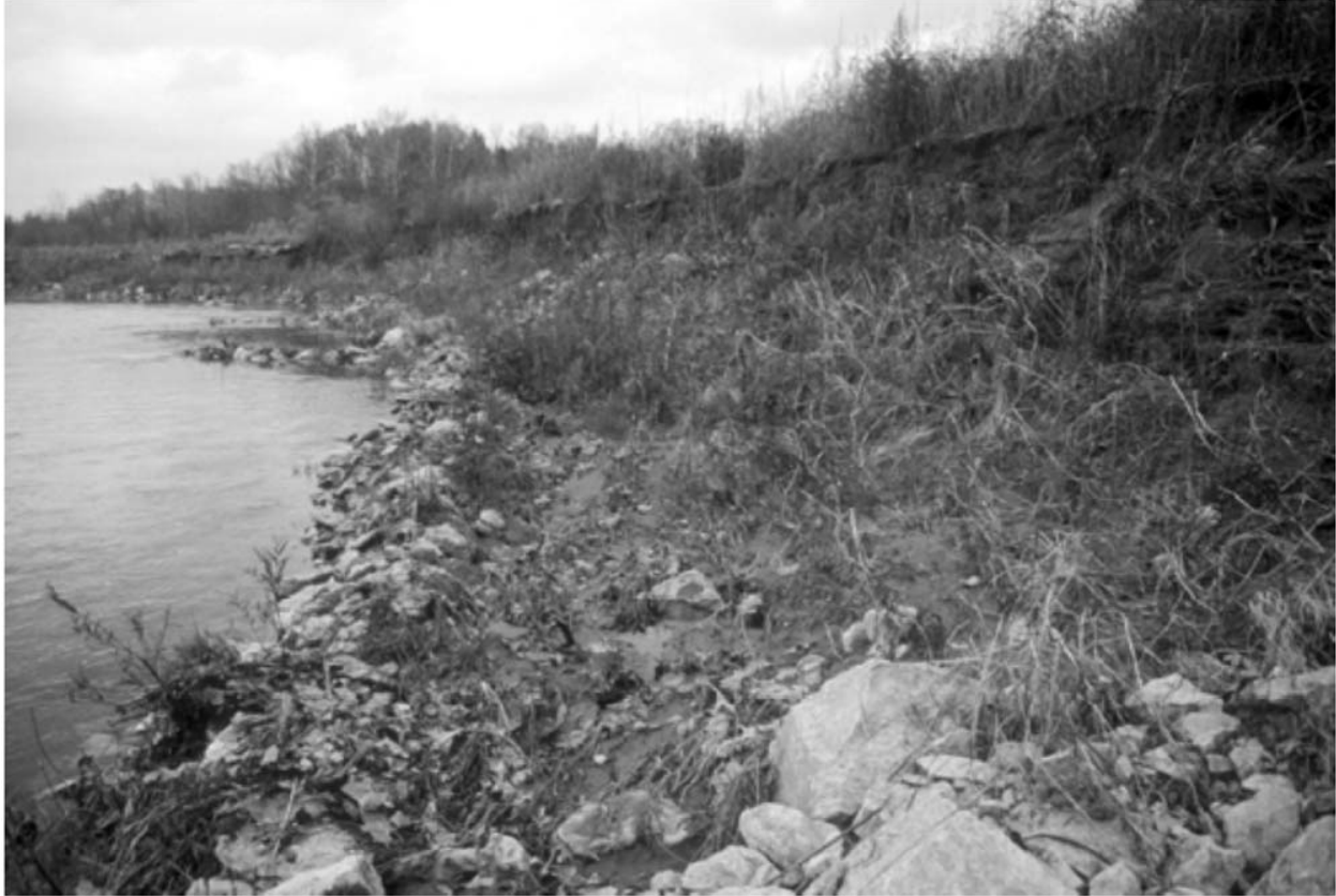
Figure 12–4. Erosion of bank face at a meander bend with bendway weirs, Big Creek, Clark County, Ill. Retreat of bank has produced a platform at the elevation of the tops of the weirs and intervening stone toe protection. Rocks in the foreground represent exposed part of the weir that was originally embedded in the bank to key the weir into the bank. A weir and its exposed key can be seen in the background. Photo used by permission from American Society of Civil Engineers. After Abad et al. (2008).
