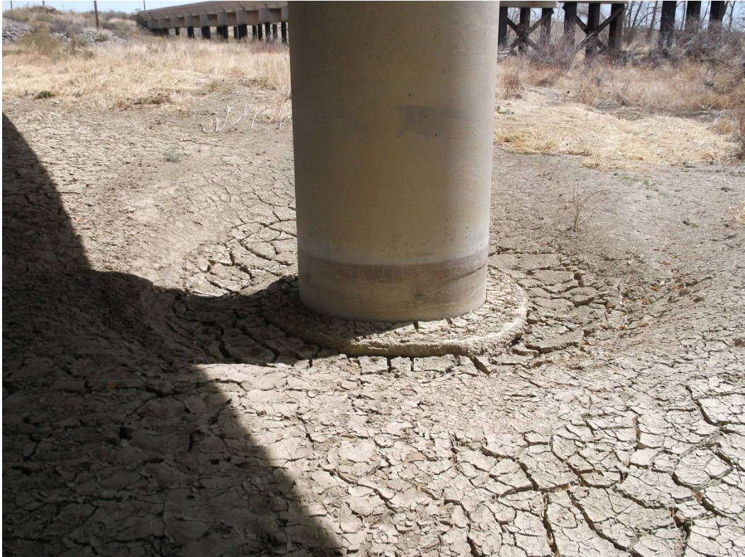
Figure 5–5. Depth of pier scour hole is partially limited by the pile cap/footing that interrupts the downward diving flow of the secondary flow pattern. This protection is lost if degradation erodes the bed and exposes the larger diameter of the pile cap to approaching flow.
