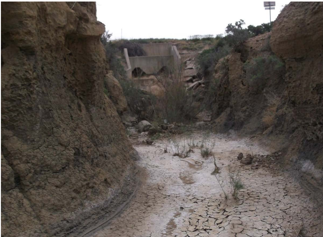
Figure 5–1. Example of channel degradation, looking upstream. Headcut migration upstream is blocked by the concrete energy dissipator that is now hung above the channel.
