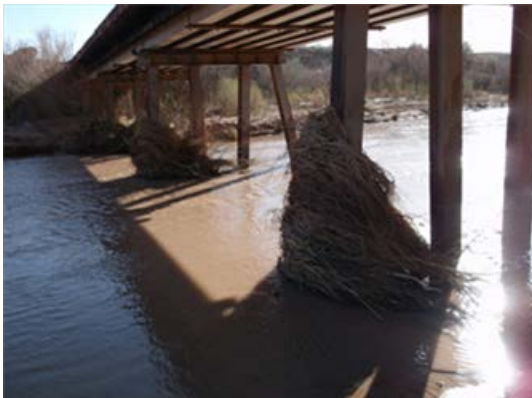
Figure 5–7. Debris caught on pile-piers of the Old Bridge from spring flows at the Little Colorado River, April 2013.
