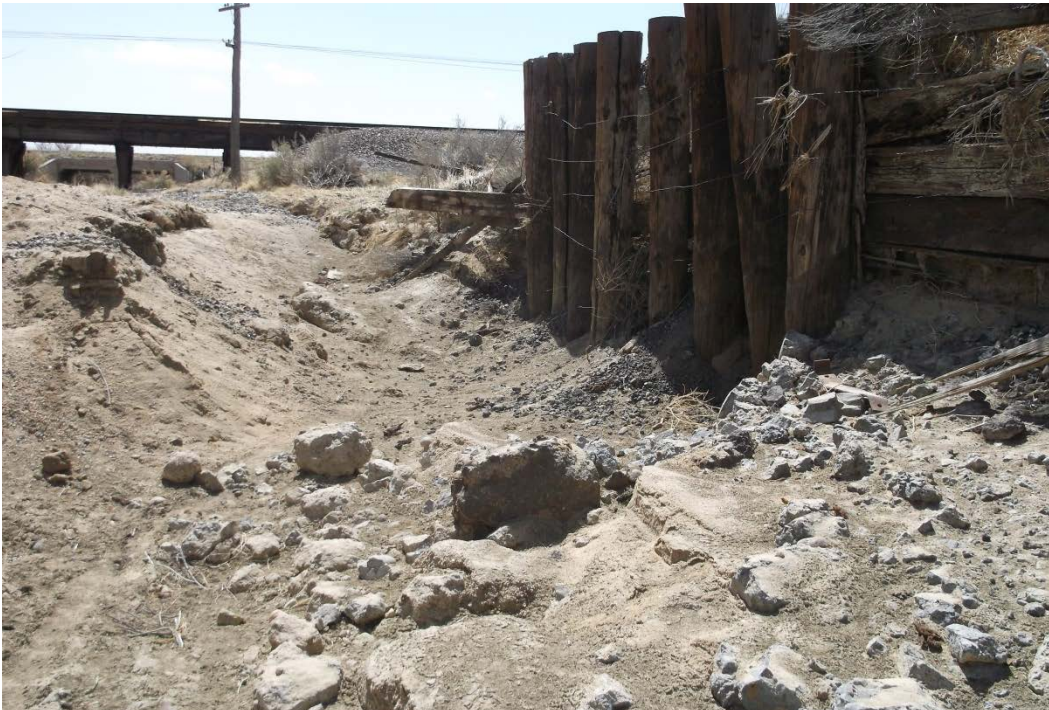
Figure 5–3. Looking downstream past scour at old railroad embankment and former bridge crossing, and towards a more recently constructed railroad embankment and timber bridge. Scour may be the result of contraction and abutment scour.
