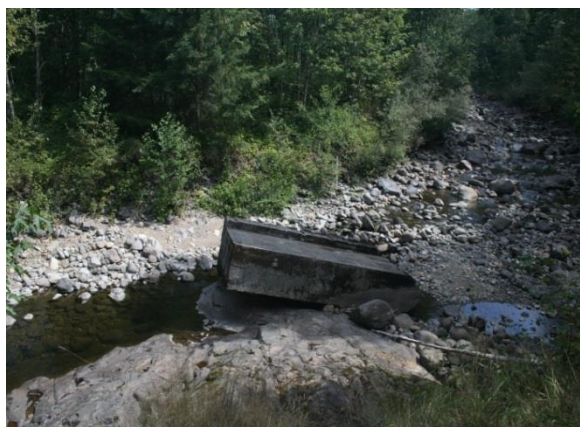
Figure 1-16. Removal of Wood Leads to Channel Incision, Converting Alluvial Pool-Riffle Channels to Bedrock and Damaging Habitat and Infrastructure, Such as this Bridge Failure in the Mashel River, Western Washington
