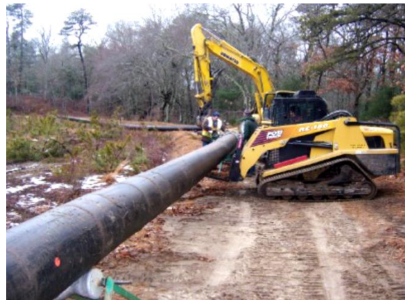
Figure 8-3. Diversion of a Small Stream Around a Construction Zone Through Plastic Pipe
