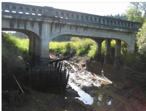
Figure 2-9. Bridge Improvements Done to Improve Wood Conveyance as Part of a Stream Restoration Project (State Route 7 over Ohop Creek, near Eatonville, Washington)
