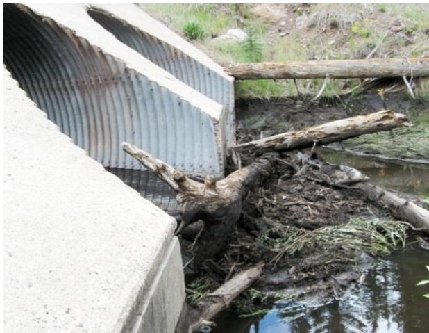
Figure 5-14. Wood Inhibiting the Flow of Water through a Culvert under Highway 4 Following the Las Conchas, New Mexico Fire (2011)
