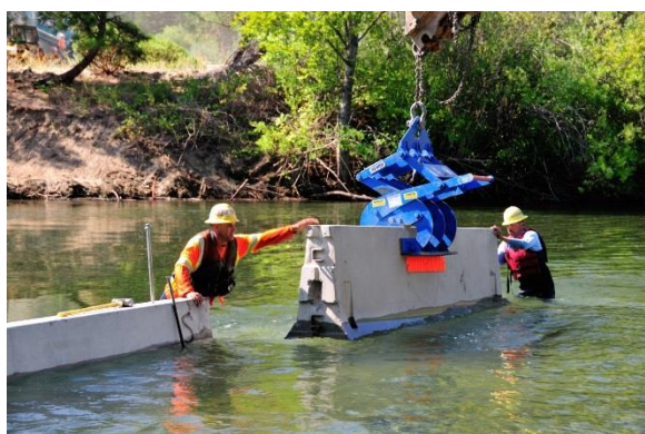
(a) Wet but controlled conditions used to isolate turbidity impacts in work zone from main channel. (b) Highway traffic barriers being used to construct a temporary isolation cell prior to wood placement. Photos by Ken DeCamp.
