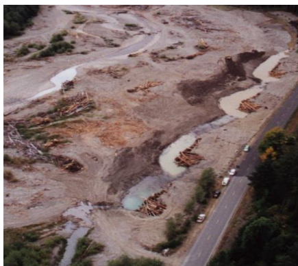
Photo e. Series of ELJ flow deflectors constructed in 1999, Cispus River, Washington (Tim Abbe).
