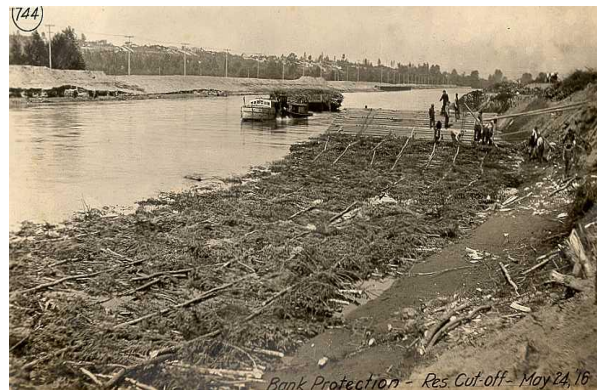
Photo b. Placement of cedar brush mattress along toe of Puyallup River North Levee, May 24, 1916 (photo courtesy of Pierce County, Washington).
