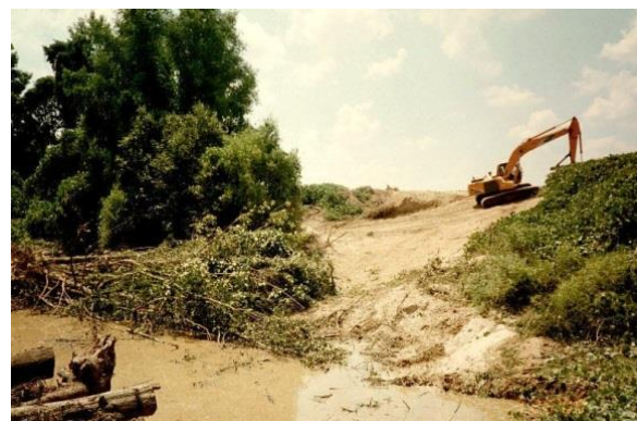
Figure 6-16. Construction of Temporary Ramp for Access to Channel for Large Wood Structure Construction in Little Topashaw Creek, Mississippi
