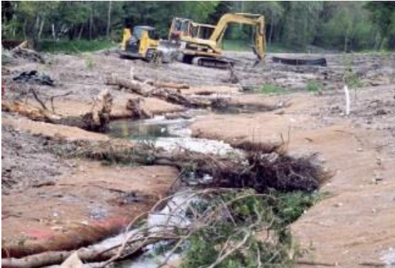
Photo i. Headwater or small perennial stream construction can use wood scaled appropriately to provide overhead cover and bank stability that can last 100 years or more (Photo by Inter-Fluve).
