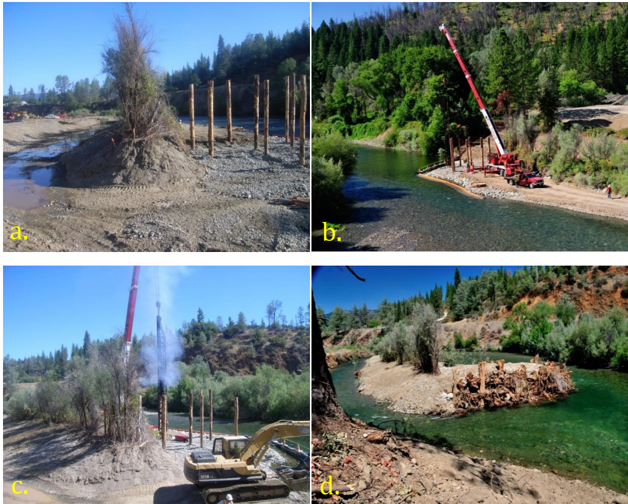
Figure 8-12. Sequence for Constructing Large Wood Structure With Vertically Driven Piles Used to Secure the Structure
