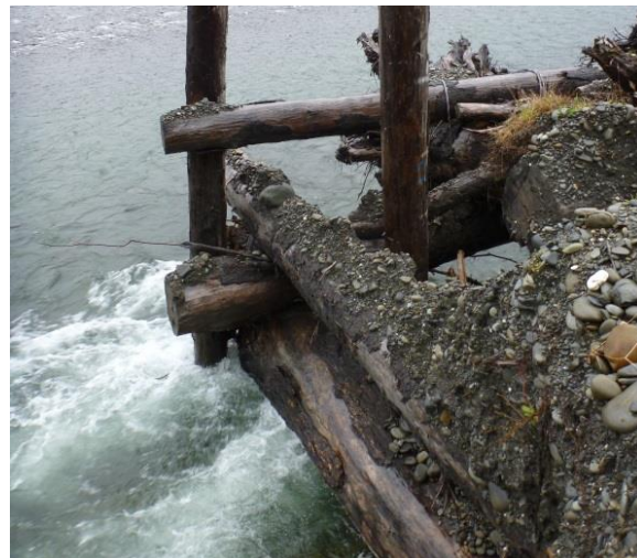
Figure 7-2. Scour Undermining Downstream Corner of an ELJ on Upper Quinault, Washington
