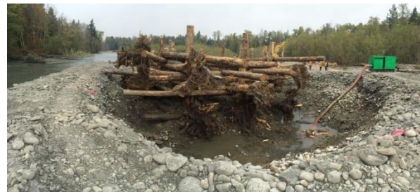
Figure 2-7. Excavation and Dewatering During Construction of an Engineered Logjam in Elwha River, Washington
