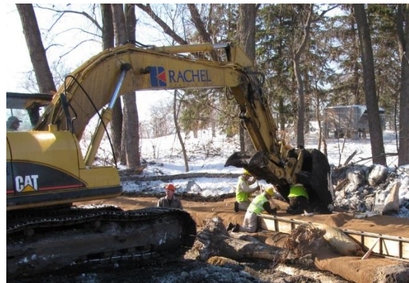
Figure 8-15. Construction Laborers Work to Secure Fabrics Around Large Wood Toe Placements on the Outside of a Meander Bend in a Shallow Channel
