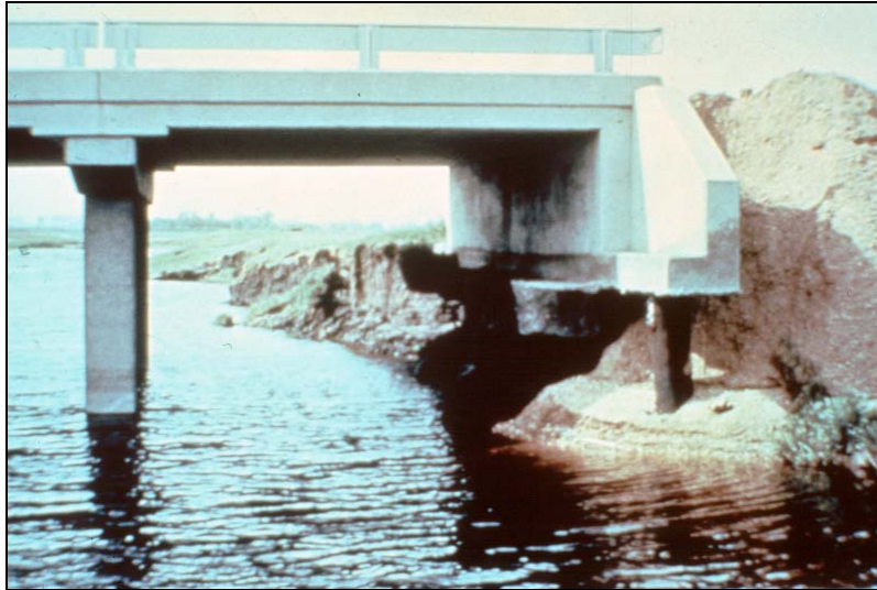
Figure 8.2. Scour of bridge abutment and approach embankment.
