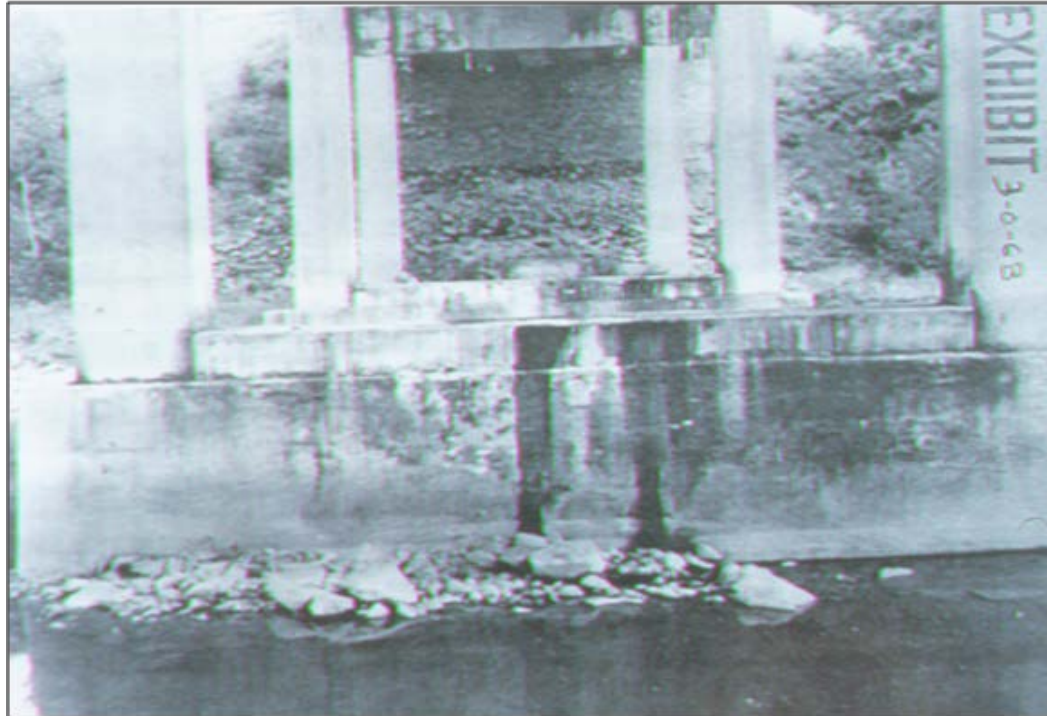
Figure 10.2. Photograph of riprap at pier 2, August 1977 (flow is from right to left).
