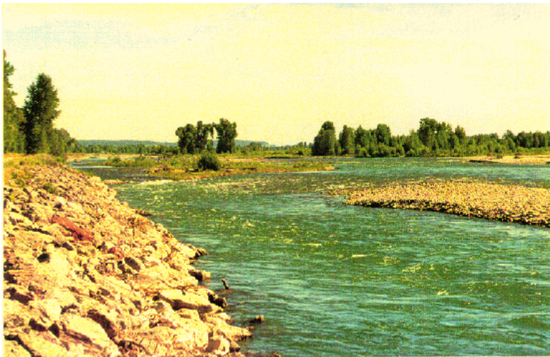
Figure 3.25 Erosion Generated by Impinging Flow
