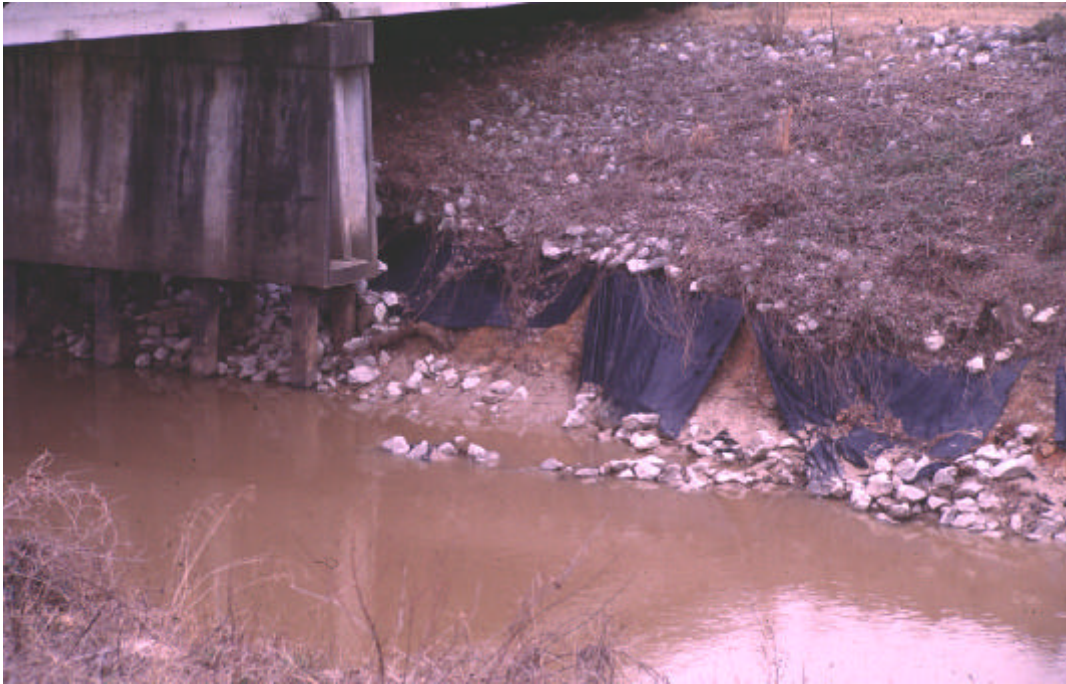
(c) Damage to Infrastructure
