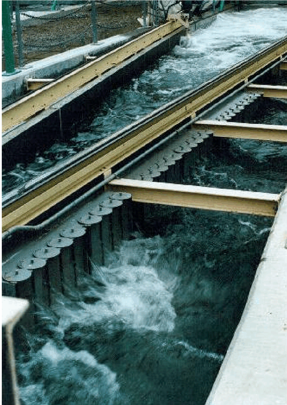
Figure 42.—Vertical van-type adjustable baffles behind Red Bluff flat plate screen.
