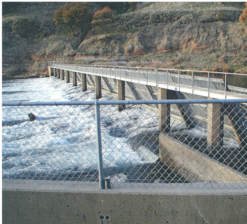
Figure 130.—Nimbus Dam bar rack barrier, American River, near Sacramento, California. (Nimbus Fish Hatchery).
