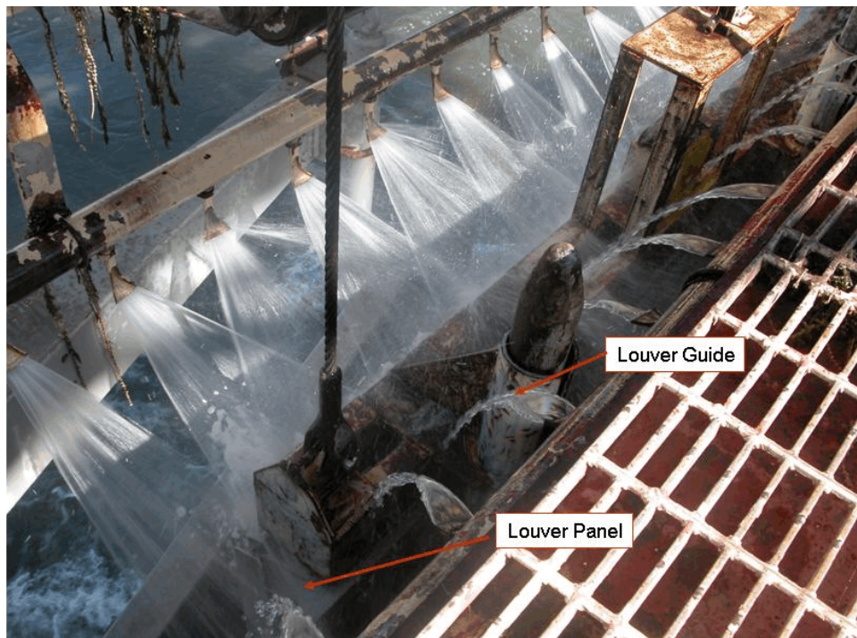
Figure 96.—Spray bar used to clean louvers at Tracy Fish Collection Louvers (downstream spray bar not operating).
