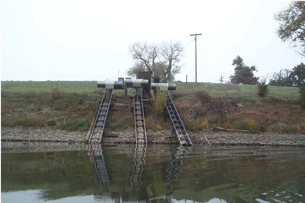
Figure 16.—Installation showing three raised retrievable cylinder screens – Davis Ranches Site #1, California (intake screens incorporated).
