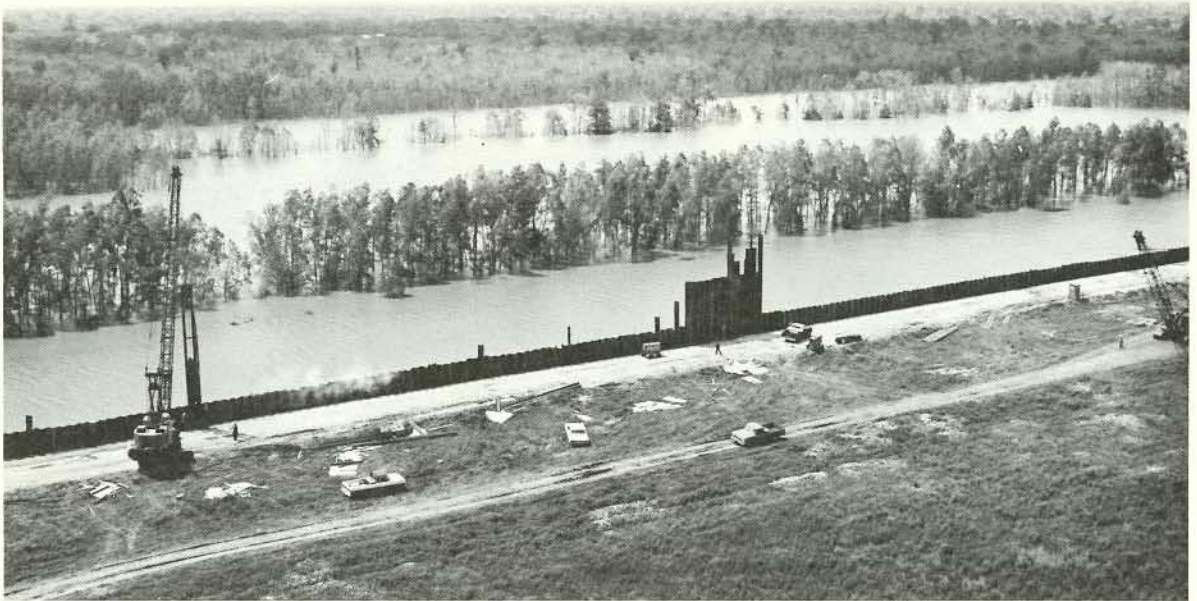
Steel sheet piling used north of Morgan City, Louisiana, East Atchafalaya Basin protection levee
