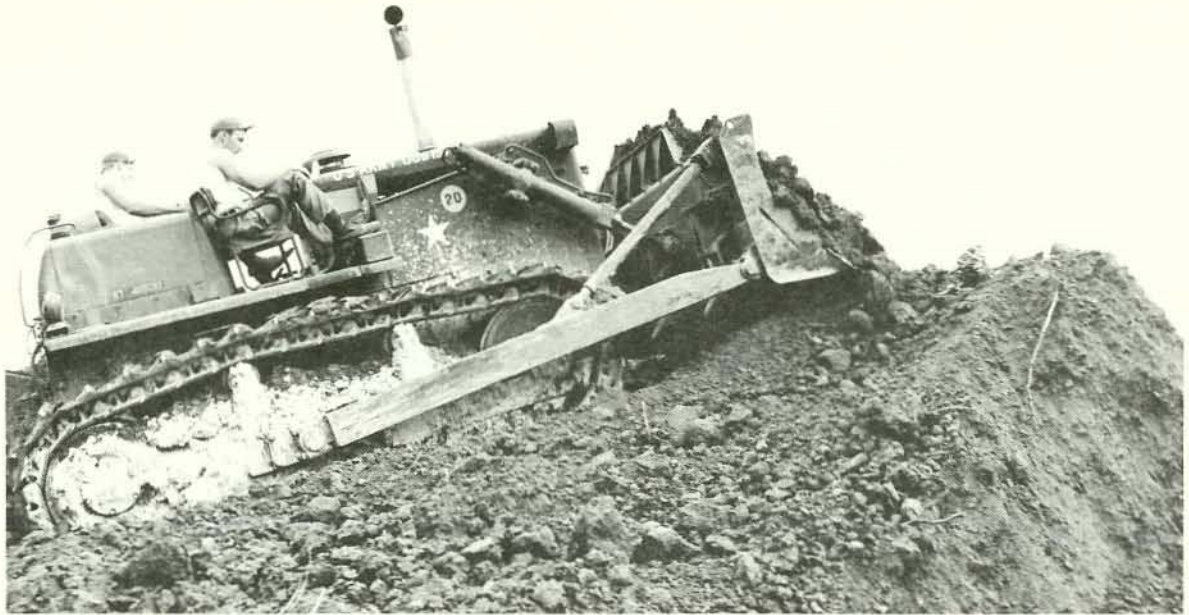
Bulldozers operated by 62d Engineer Battalion were effective in levee-raising operations, Morgan City, Louisiana
