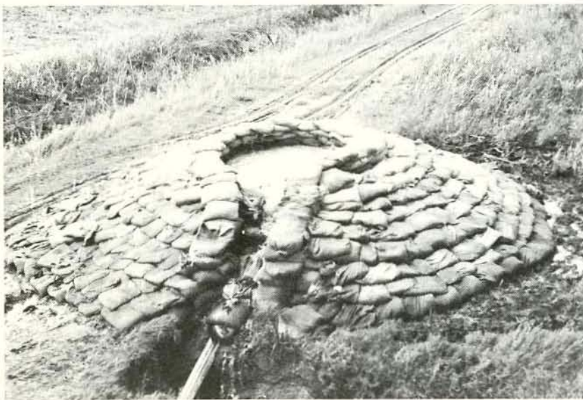
Typical example of a sand boil, ringed with sandbags to create enough head to slow the flow
