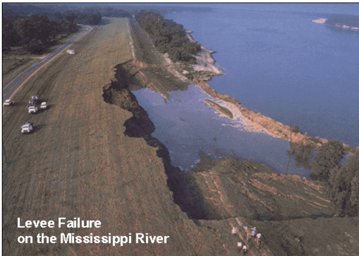
Figure 14: Levee failure on the Mississippi River during the 1993 flood event Source: U.S Army Corps of Engineers
