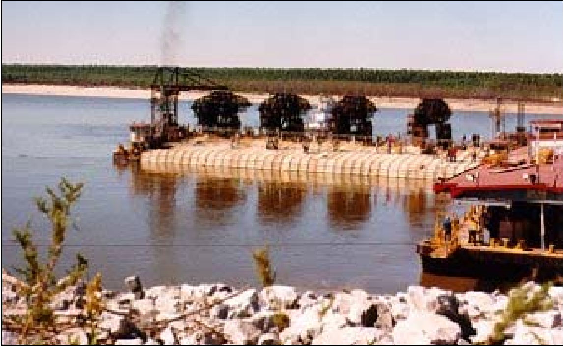
Figure 20: Articulated concrete mattress installation in the upper Mississippi River Source: U.S. Army Corps of Engineers
