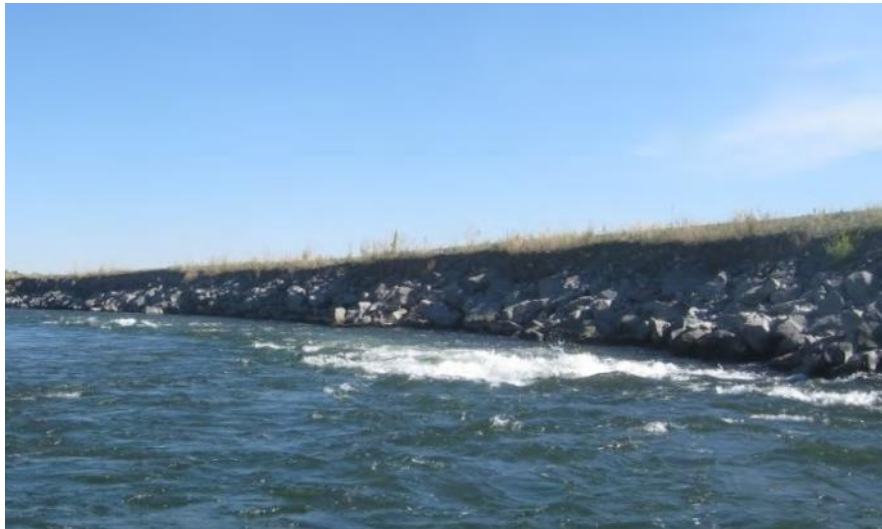
Figure 16 - View downstream of intercepted trenchfill revetment; local turbulence is from launched rock (Boyd, 2010)
