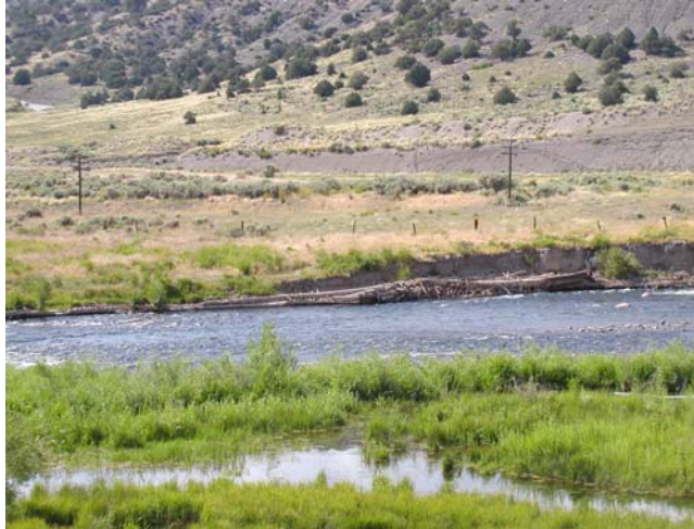
Figure 4.127: Bank failure upstream of Wolcott.
