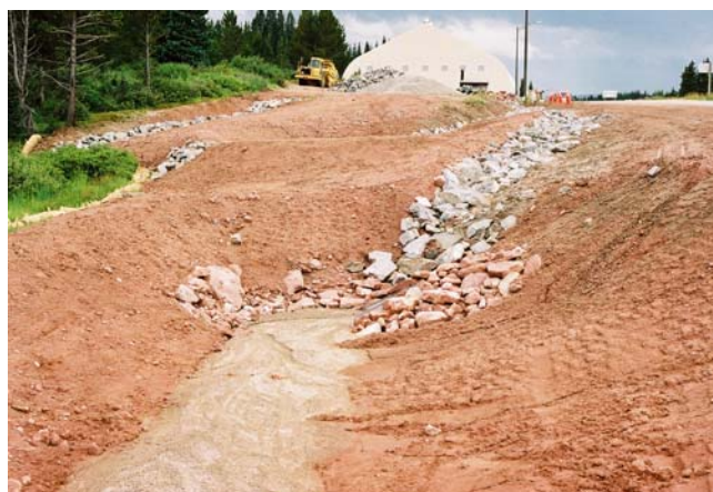
Figure 4.136: Sediment basins along Vail Pass for trapping traction sand.
