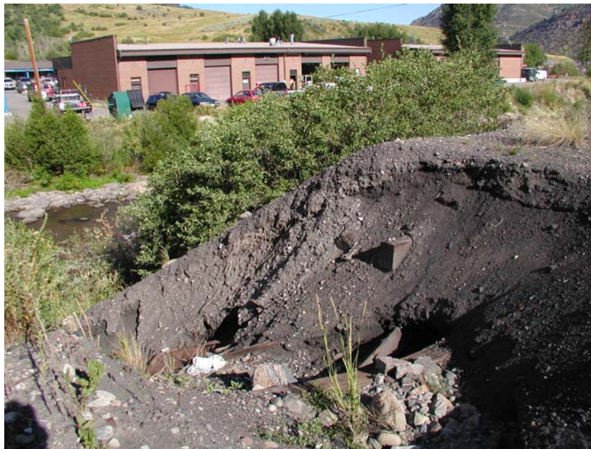
Figure 4.107: One of the larger erosion features along the railroad yard downstream of Minturn.
