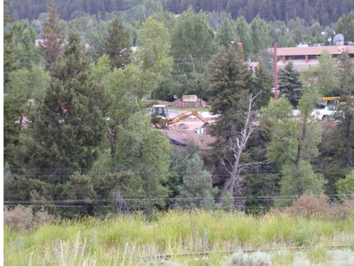
Figure 4.111: Construction in Eagle-Vail with poorly functioning silt fence.
