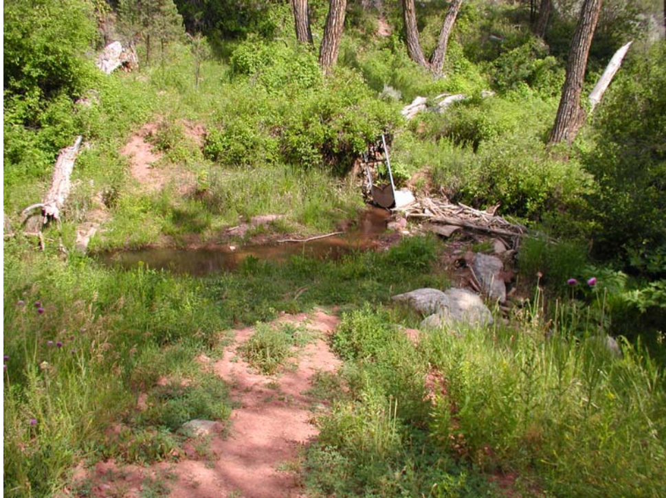
Figure 4.147: Poorly functioning diversion structure Eby Creek.
