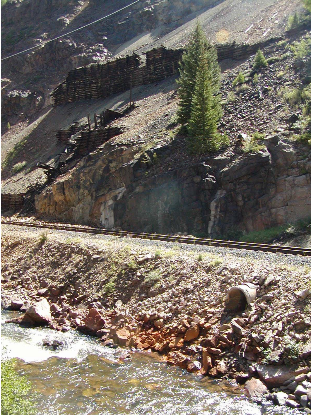
Figure 4.95: Culvert that delivers metal contaminated water from a leaking mine adit located upstream of the Superfund site. Notice cribs in background.
