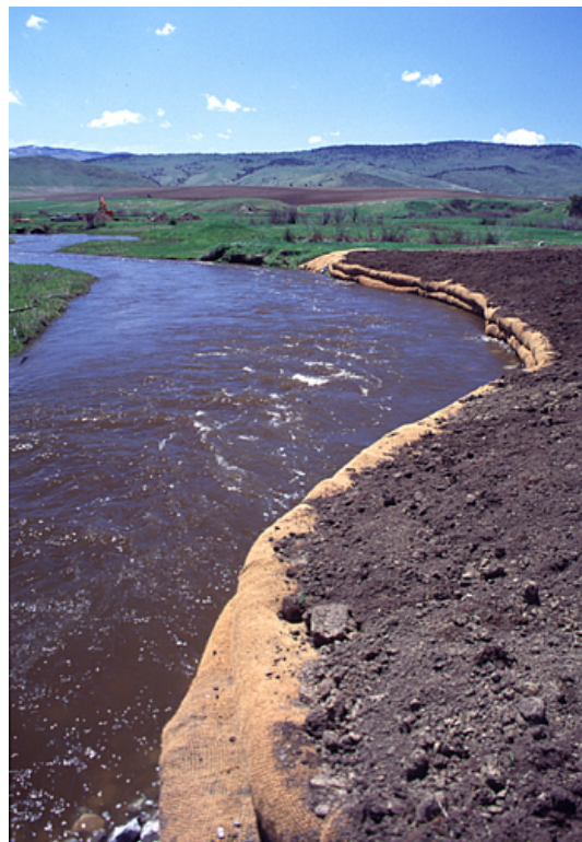
Figure 25: Typical fabric lift installation. Top left shows original bank; top right shows first lift being placed over the gravel platform. Bottom picture shows soil placement over the last lift, prior to seeding.
